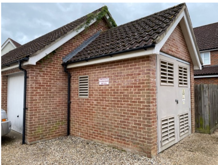
Figure 105: Utilities housed in a unit in-keeping with surrounding dwellings. Mulbarton, Norfolk. Source: own.
