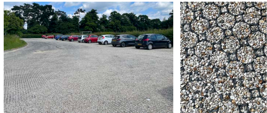
Figure 66: Permeable surfaced for car park. Community car park at Willow Centre, Cringleford, Norwich. Source: own.
