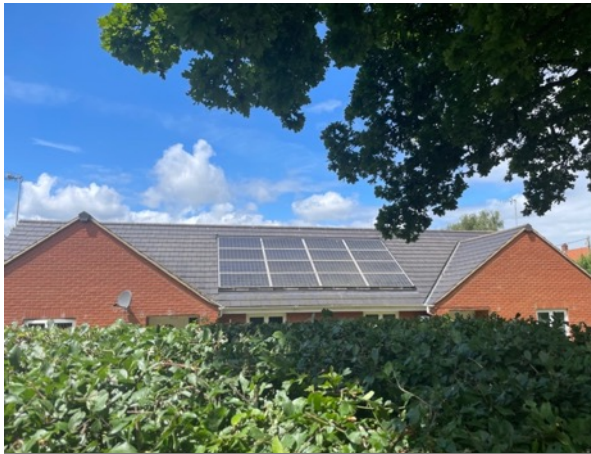
Figure 101: Solar panels incorporated into the roof. Green Lane West, Rackheath. Source: Own.
